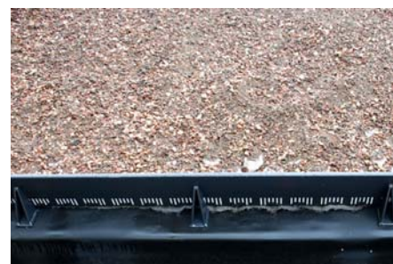
The shear forces exerted by the green roof build-up are being derived into the roof structure via a slotted eaves profile and shear brackets.
