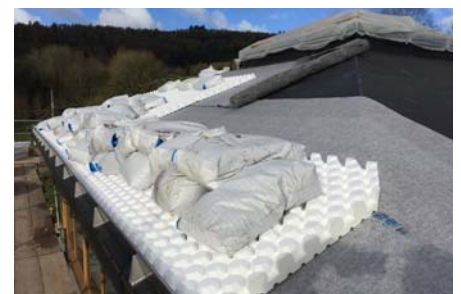
... the eaves profiles TRP 140 were set loose onto the protection and water retention mat BSM 64; Floraset® FS 75 elements were laid out on the entire roof surface.
