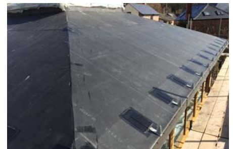
The TSH 100 support brackets were installed and sealed in line and parallel to the eave ...
