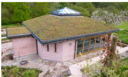
Even the roof of the entrance area was greened, however, Floradrain® FD 25-E was used as a base.
