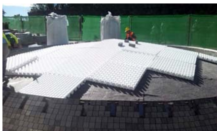
The entire surface of each planter was covered first with the protection mat and then with the drainage elements. The Floraset® elements were cut to shape to follow the curves of the surfaces.
