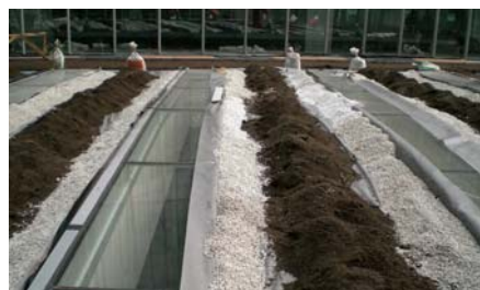
The system substrate and the gravel (for the edges) are distributed evenly all over the roof surface.
